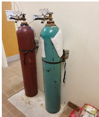
Cylinders secured to a wall.
